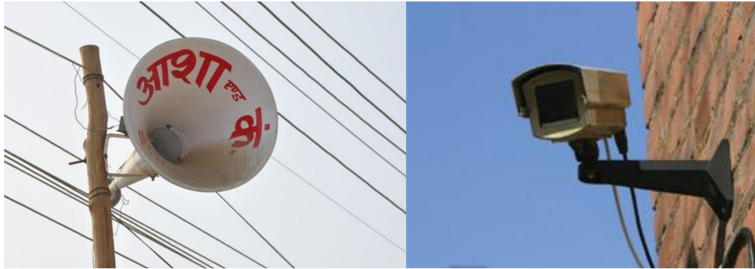
Figure 8: Public Announcement System and CCTV Camera
